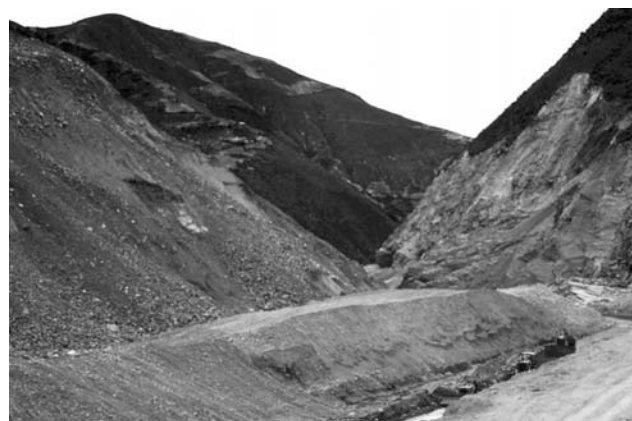
Figure 19 - Excavation of a new channel in the landslide mass after the May 1 st , 1993 overflow. The unstable left slope that needed a stabilizing scheme can be observed
