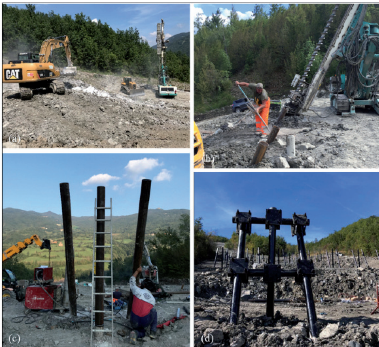
Fig. 5 – Field views of the main MTS construction phases. LEGEND: (a) working site preparation with lime-treatment of the surficial layer of the embankments; (b) underground micropiles drilling and installation; (c) aboveground micropiles welding; (d) tripods completed with connection beams and plates
