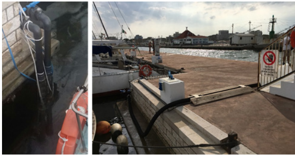
Fig. 9 - Two pictures taken during the on-field tests. The two submersible pumps (left) and the passage of temporary supply piping.
