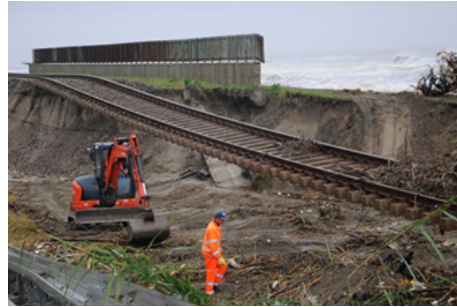
Fig. 9 - The suspended railway tracks at Bruzzano Zeffirio following the event of 31 st October-2 nd November.
