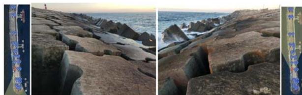
Fig. 7 - Systematic photos took during visual observation in the Sines west breakwater (Point 27).
