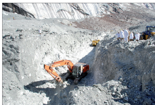
Fig. 14 - Heavy equipment excavating human remains and the artificial spillway. Photo courtesy of ISPR. Note the compacted debris consisting of ice and crushed rocks. Blasting efforts were not successful
