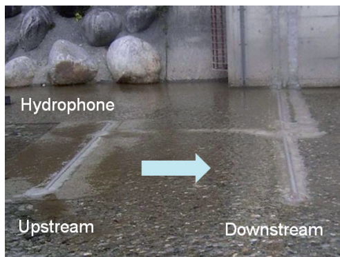
Fig. 3 - Hydrophone in Bouzudaira Sabo Dam, Yotagiri River, Japan
