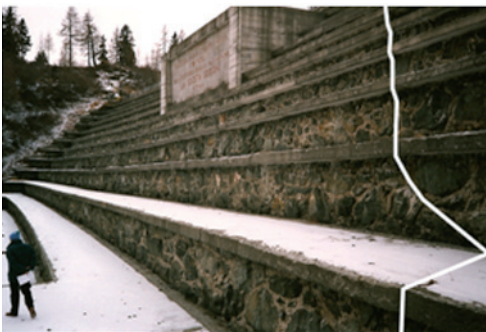
Fig. 5 - Down stream abutment of Alpe Cavalli dam with indication of the observed vertical crack
