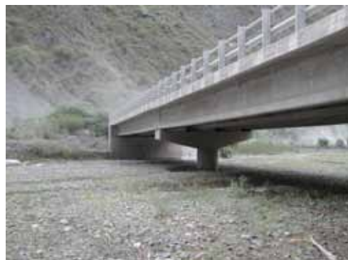
Fig. 7 - The bridge located upstream the confluence of Río Candado with Río Toro, frequently affected by floods during the rainy periods
