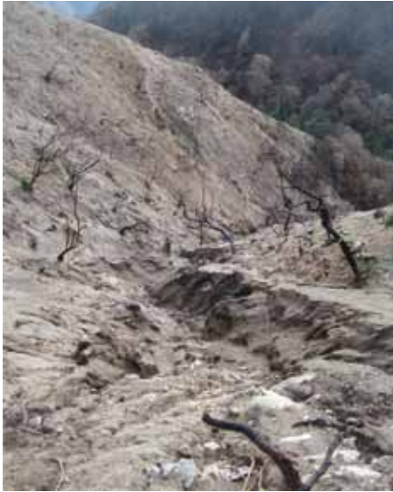
Fig. 7 - Photograph of channel erosion after the 18 Jan. 2010 storm (Storm 3). Geologist for scale in center of photo. Much of the channel bed in the foreground is bedrock
