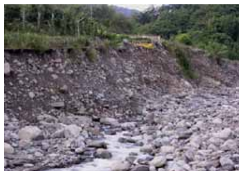
Fig. 6 - (a) River bank erosion by debris flows in Aiyuzih creek
