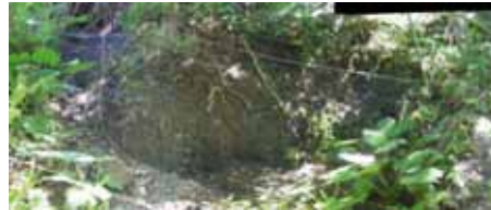
Pic. 4 - Landslide deposition on right bank hill
