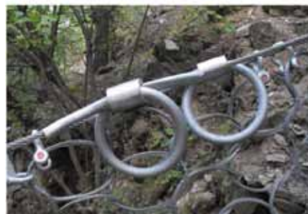
Fig. 14 - ROCCO® ring net and the braking elements, in the Portainé Torrent after the 22 nd July event
