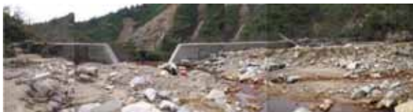
Fig. 6 - Sediment deposition caused by the upstream check dam on the Tsurugi River (View from upstream to downstream direction on November 27, 2009)
