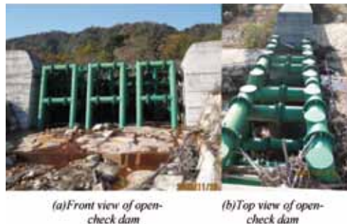
Fig. 24 - Sediment and driftwood at the downstream check dam in the Hachimandani River on November 25, 2009
