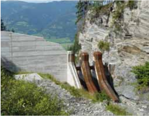
Fig. 1 - Debris breaker in the Rastetzebach torrent in Bad Hofgastein (Salzburg)
