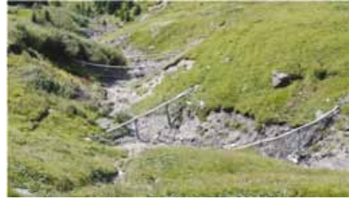
Fig. 10 - Multi-level debris flow barriers in Hasliberg region, Switzerland
