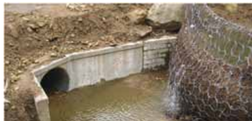
Fig. 15 - Net barrier against culvert blockage installed directly in front of a culvert, The Narrows, CA
