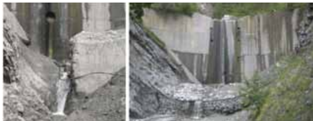
Fig. 14 - Scoured check dam base (left) and protected check dam base by a naturally filled net barrier
