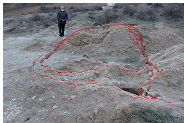
Fig. 7 - Crack initiation in loess soils due to self-weight collapse (Cheshmehli village)
