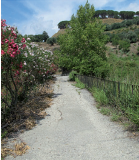
Fig. 7 - Cracks in the bituminous conglomerate on the top of the dam of the Scillupia reservoir
