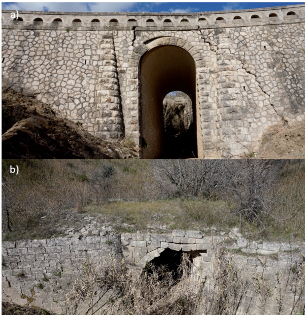
Fig. 4 - a) View of the SE side of the damaged bridge. b) Old, damaged bridge
