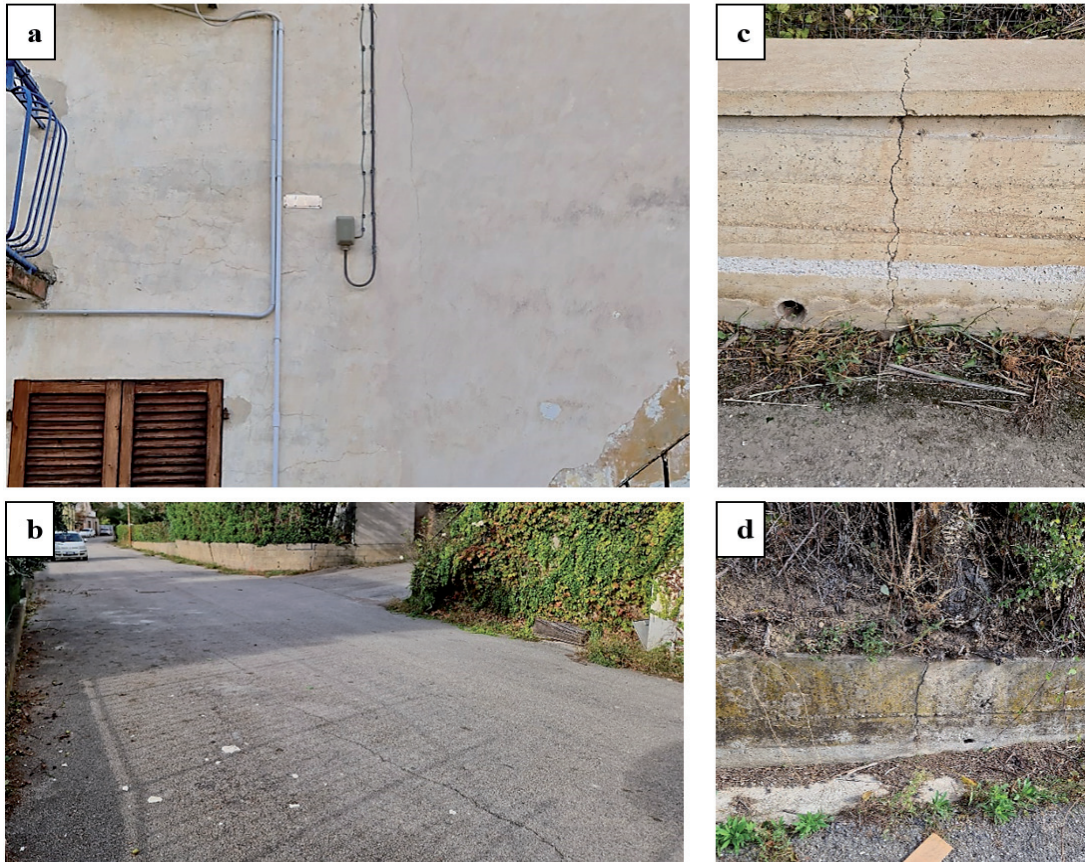
Fig. 3 - Evidence of damage, typical of landslide deformations, on the external walls of surrounding buildings (a), along the road pavement (b), and the walls bordering the road under the viaduct (c, d)
