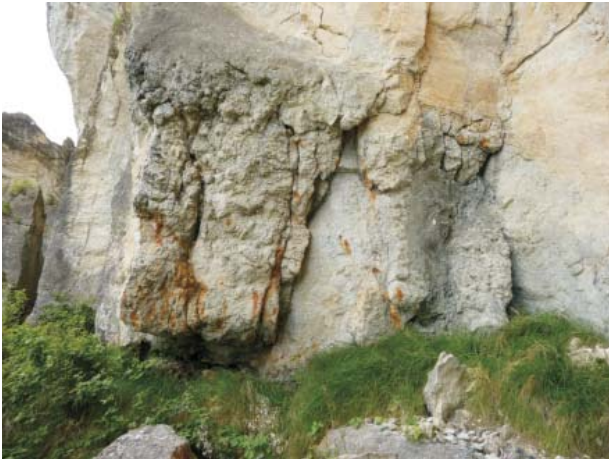
Fig. 6 - Stratigraphic boundary between AVR (hidden by vegetation) and SMN1, that is only a few meters thick
