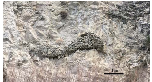
Fig. 20 - Small-block debris retained by the hexagonal metal mesh net
