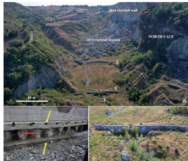
Fig. 11 - a) Aerial photo of the two first works carried out for the stabilization of the 2014 rockfall deposit along the Campone valley. Legend: 1 - the downstream structural work; 2 - the upstream structural work; 3 - the Campone stream. b) the downstream structural work was founded on large diameter piles (1) and strengthened by a double line of active nails (2 and 3); c) boulders were used to reduce the environmental impact of both structural works
