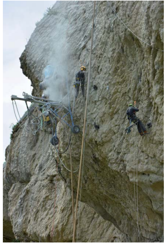
Fig. 19 - Rock drilling operations with mountaineering technique before the subsequent installation of the bars
