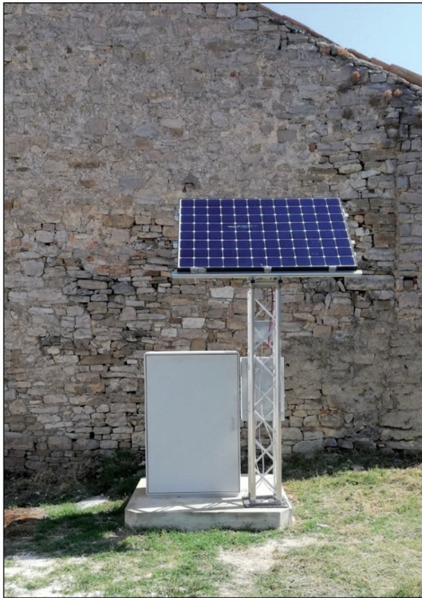
Fig. 6 - Final configuration of the Installation of the Automated Inclinator System (AIS)
