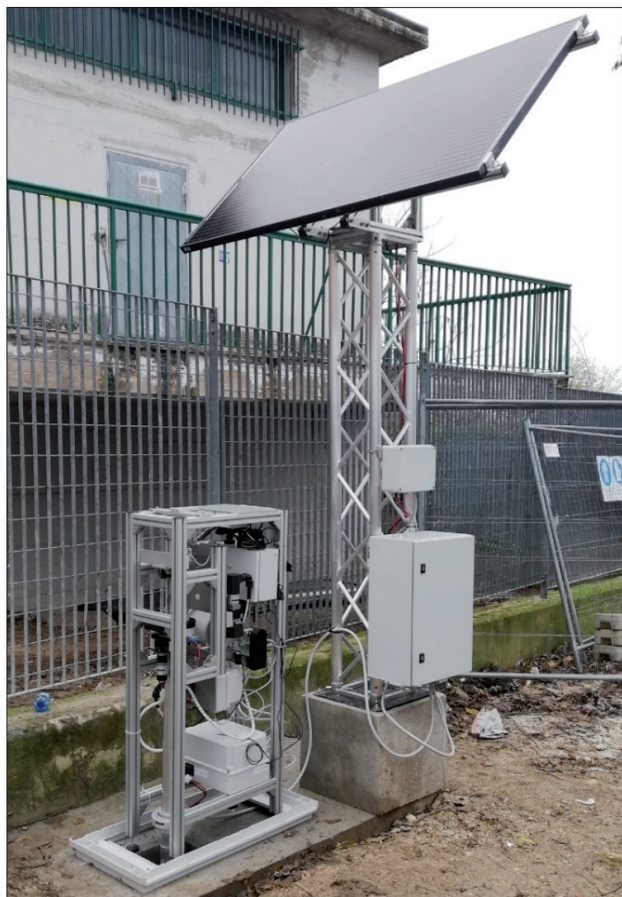
Fig. 11 - Automated Inclinerometer System with power system that include 400w solar panel and storage battery
