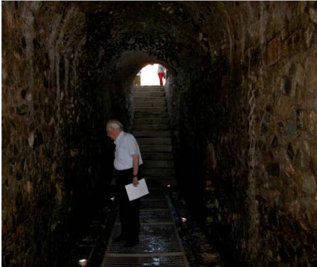
Fig. 9 - Tunnel n. 1 with the floor protected by a metallic grid and the staircase of access
