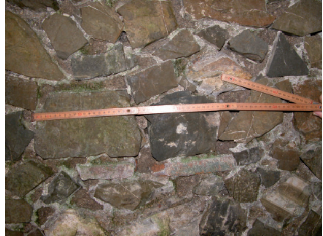
Fig. 11 - Ashlars of marly limestone and siliceous limestone cemented by gray hydraulic mortar with white calcareous inerts of the face of tunnel n. 1
