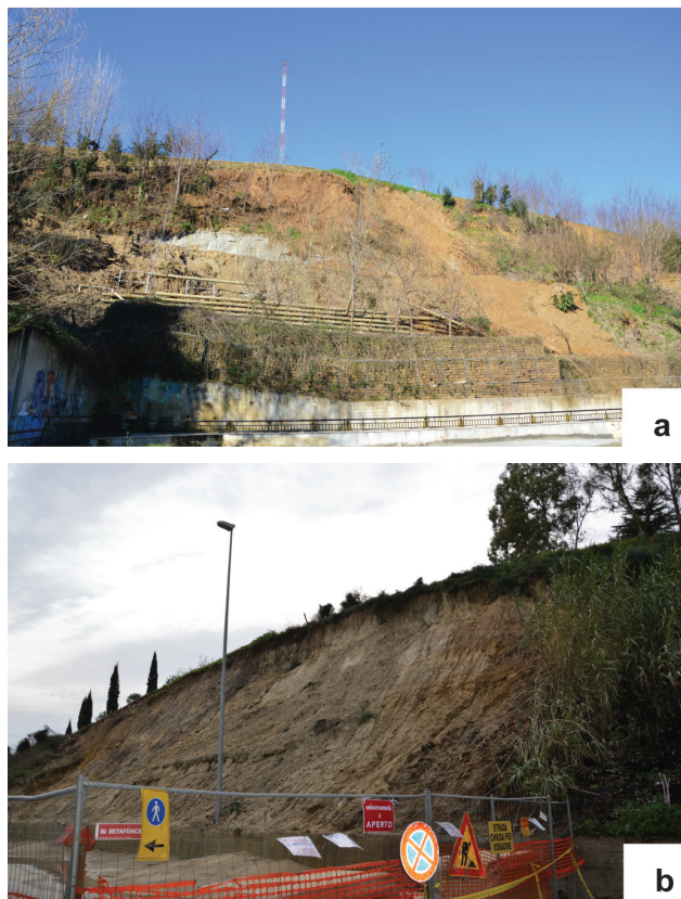
Fig. 10 - Examples of landslides triggered in Rome by the exceptional rainfall event of 31 Jan.-2 Feb. 2014: a) complex slide along Via Simone Simoni (Monte Ciocci); b) rotational slide along Via della Maglianella
